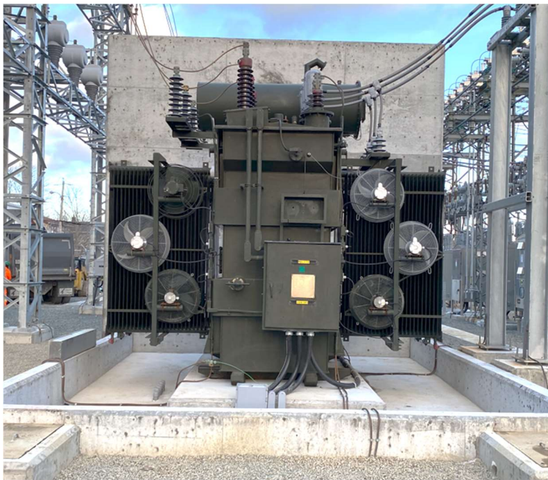
Figure E-4: Power Transformer MOL-T2.
