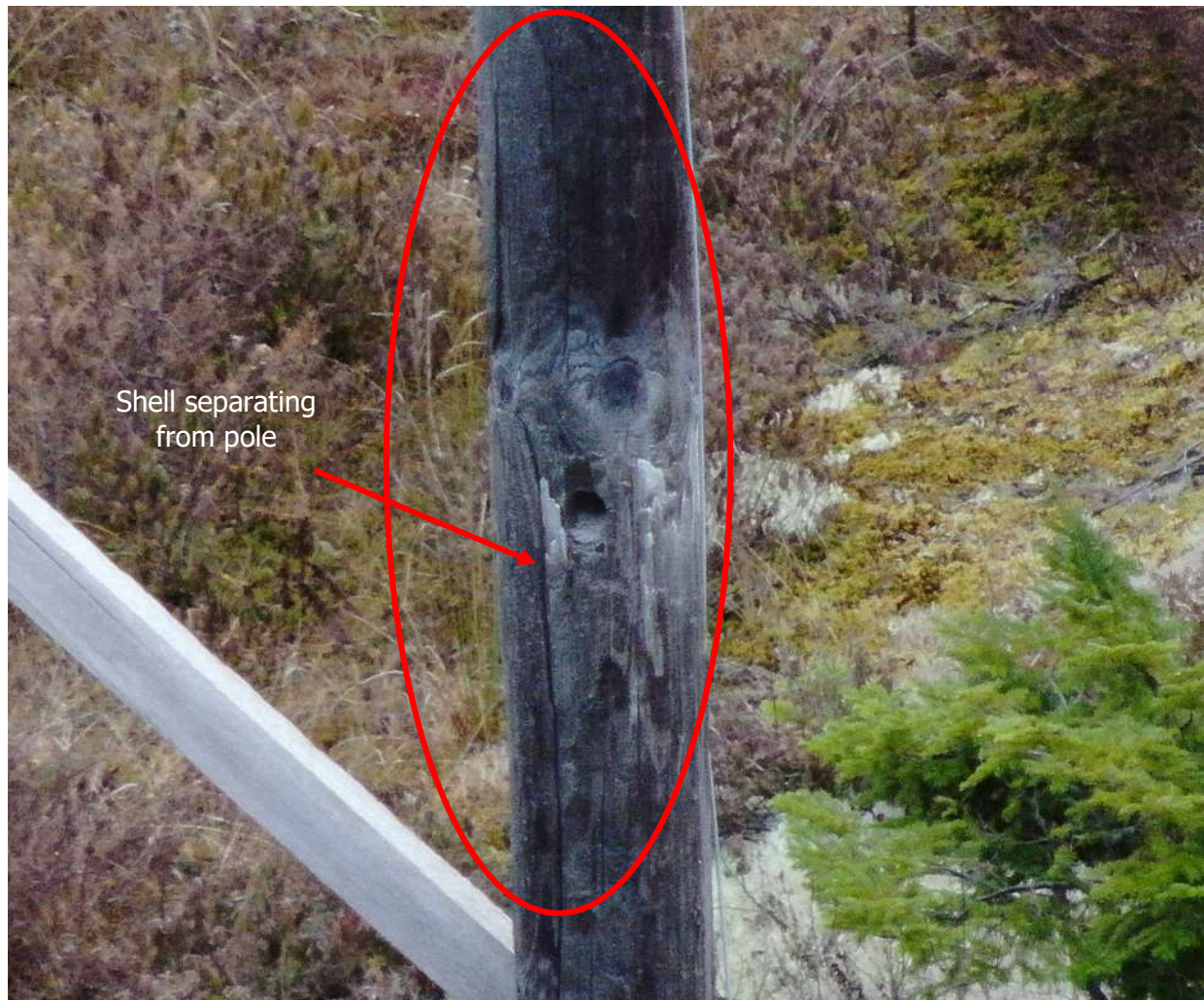
Figure 2 – Shell Separation and Woodpecker hole on 100L.
