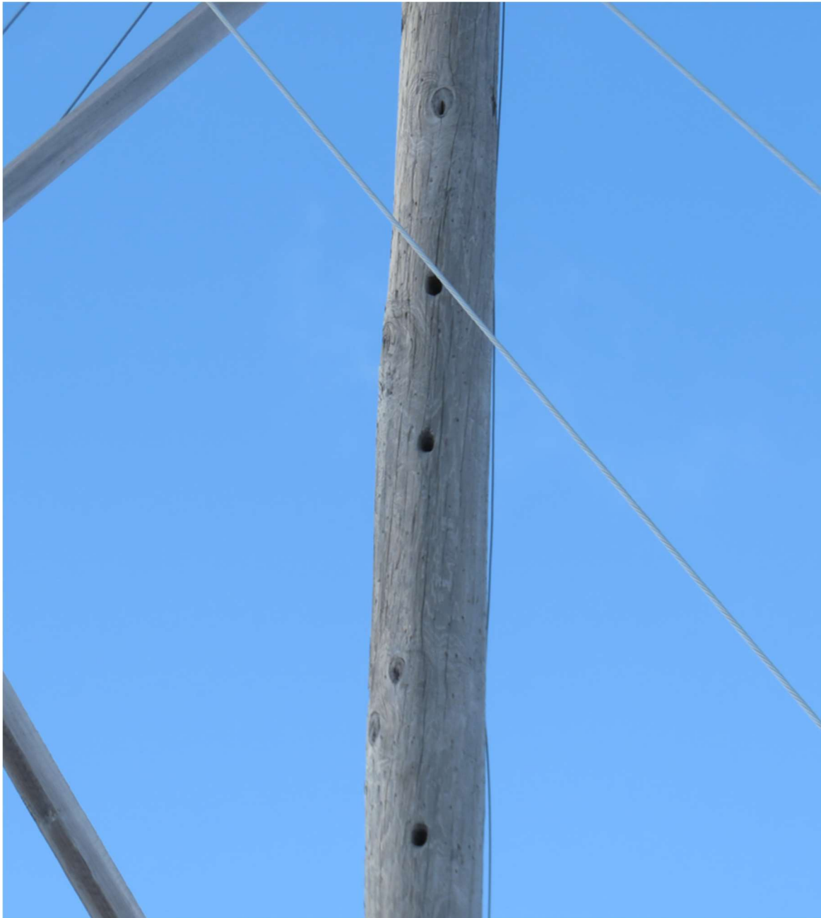
Figure 4 –Poles with Numerous Woodpecker Holes on 100L.
