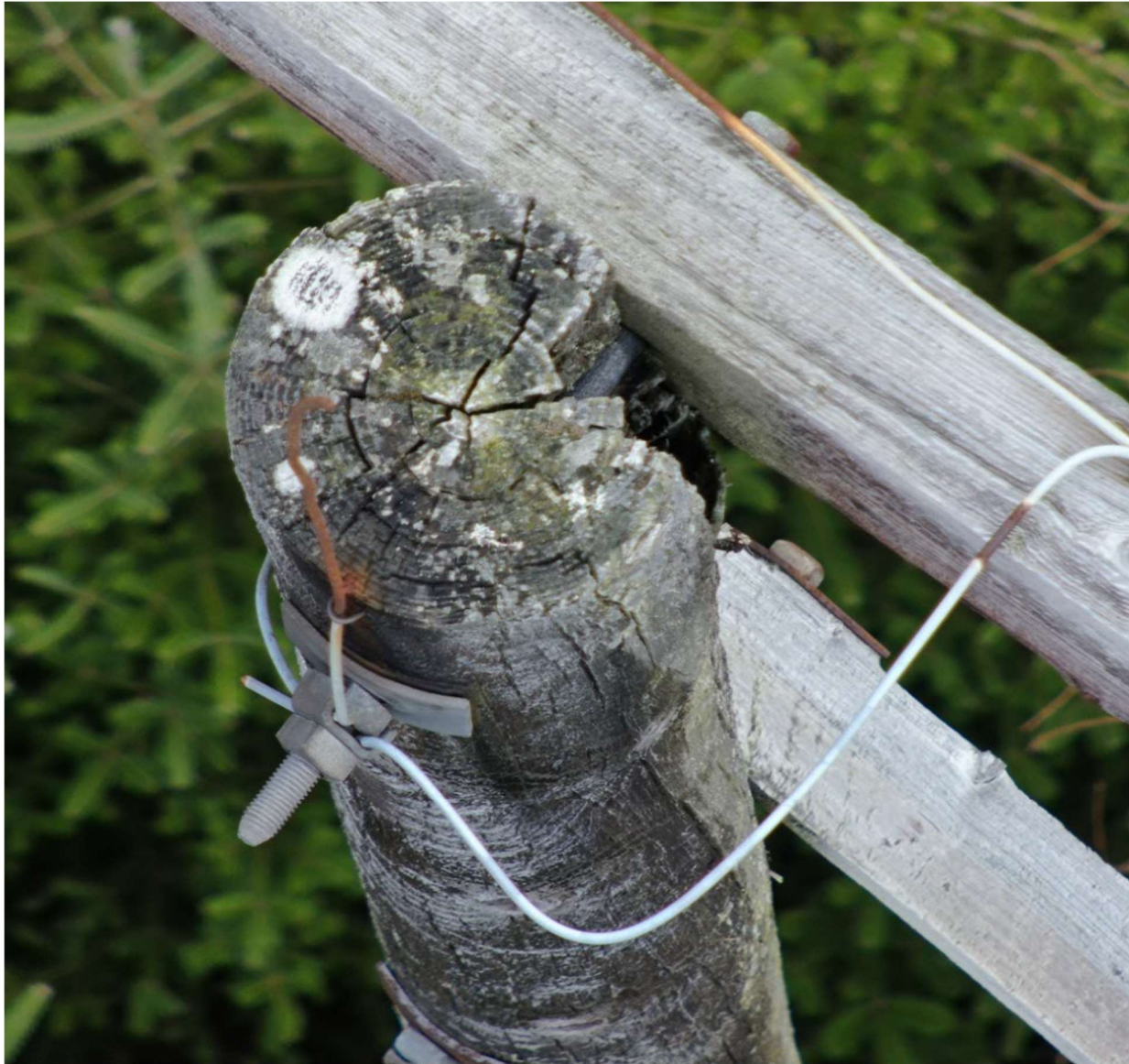
Figure 3 – Pole top Narrowing and Decay.
