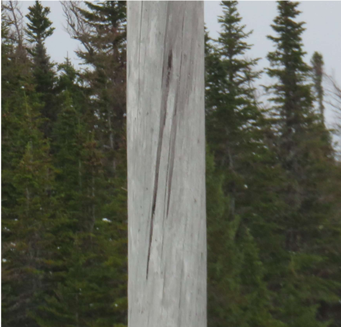
Figure B-9 – Shell Separation.
