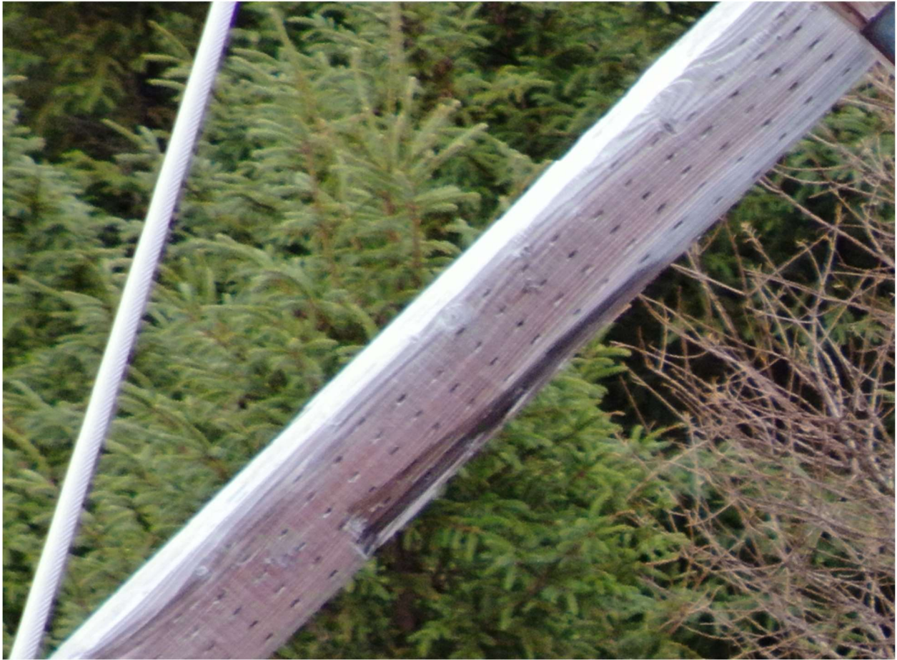
Figure B-10 – Damaged Cross Brace.
