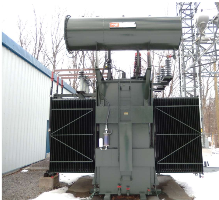
Figure E-1: Power Transformer KBR-T3.
