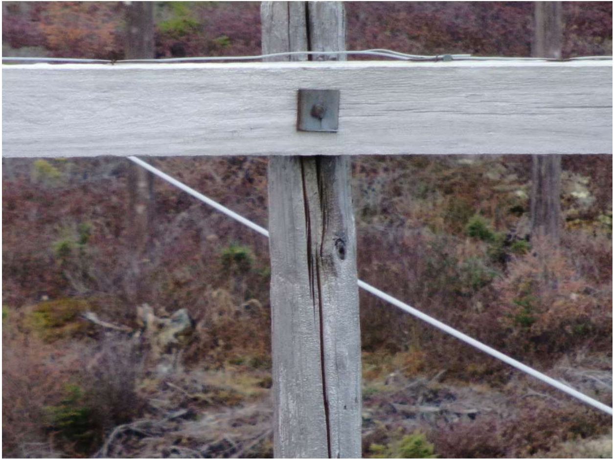
Figure B-1 – Void in Pole Top, Hollow Pole.
