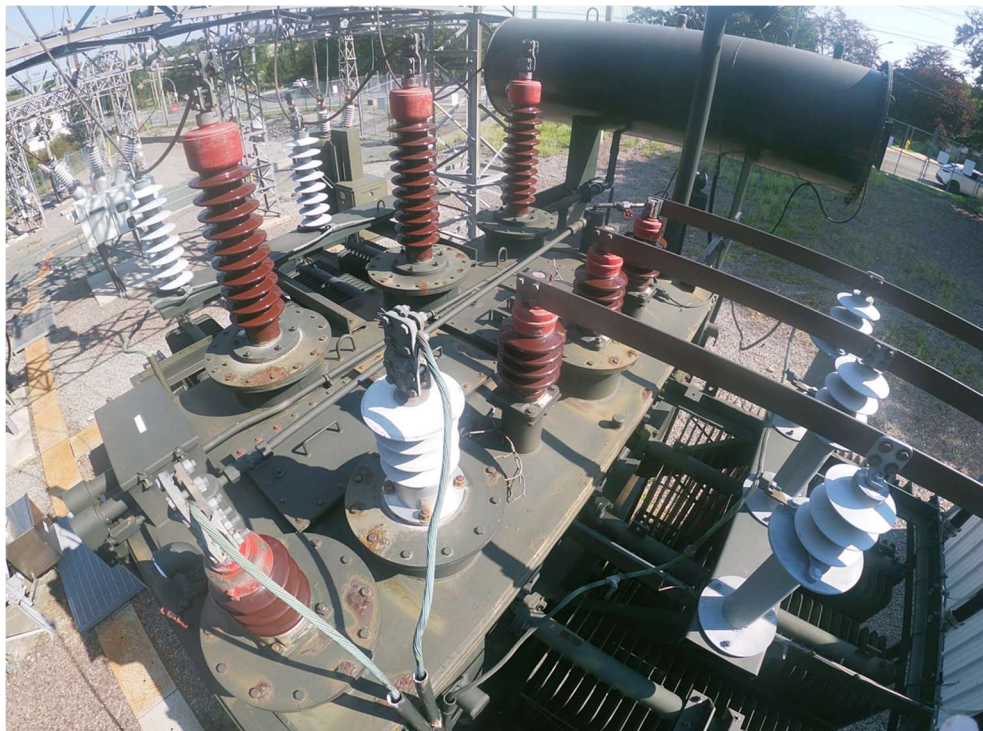
Figure E-3: Top of Power Transformer KBR-T3.
