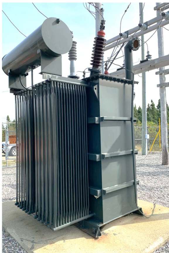
Figure A-4: GPD-T1 Power Transformer.
