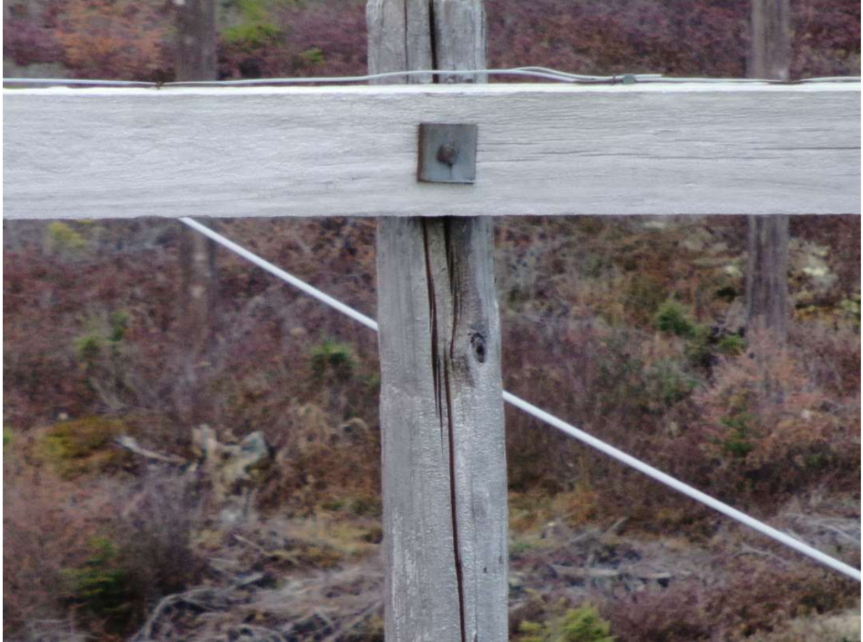
Figure B-3 – Severe Splits in Pole through Cross-Arm Bolt Locations.
