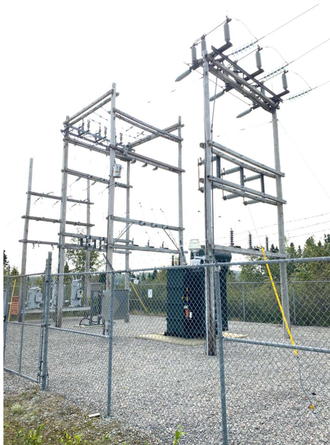
Figure A-1: GPD Substation.
