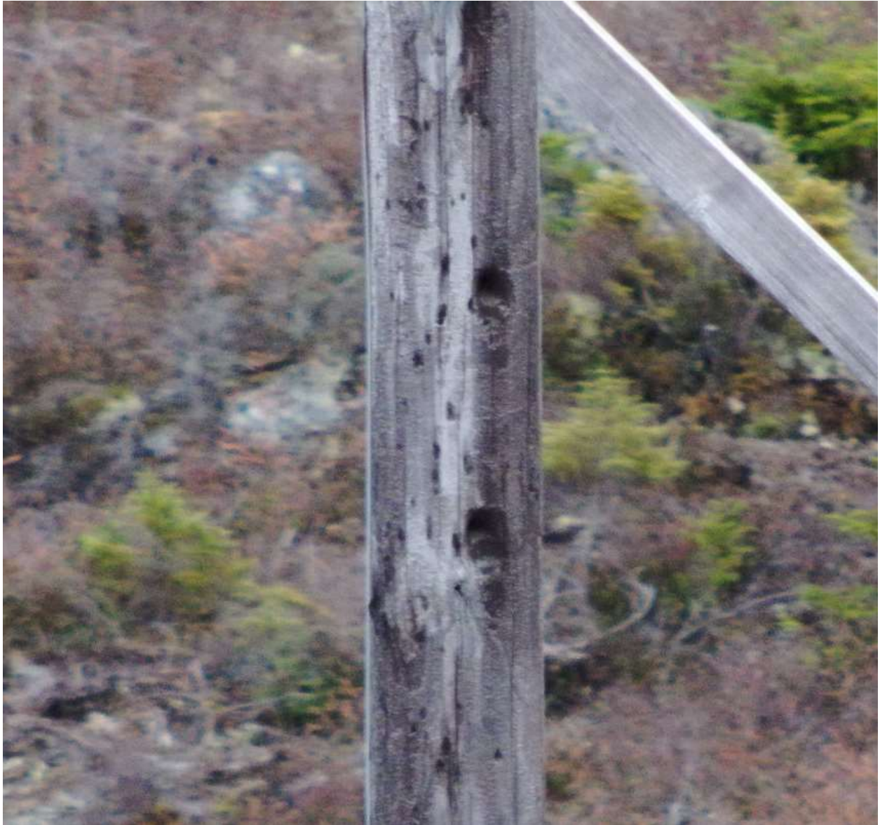
Figure B-8 – Woodpecker Holes, Hollow Pole.
