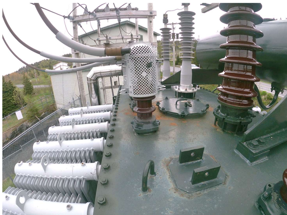
Figure E-8: Top of Power Transformer MOP-T1.
