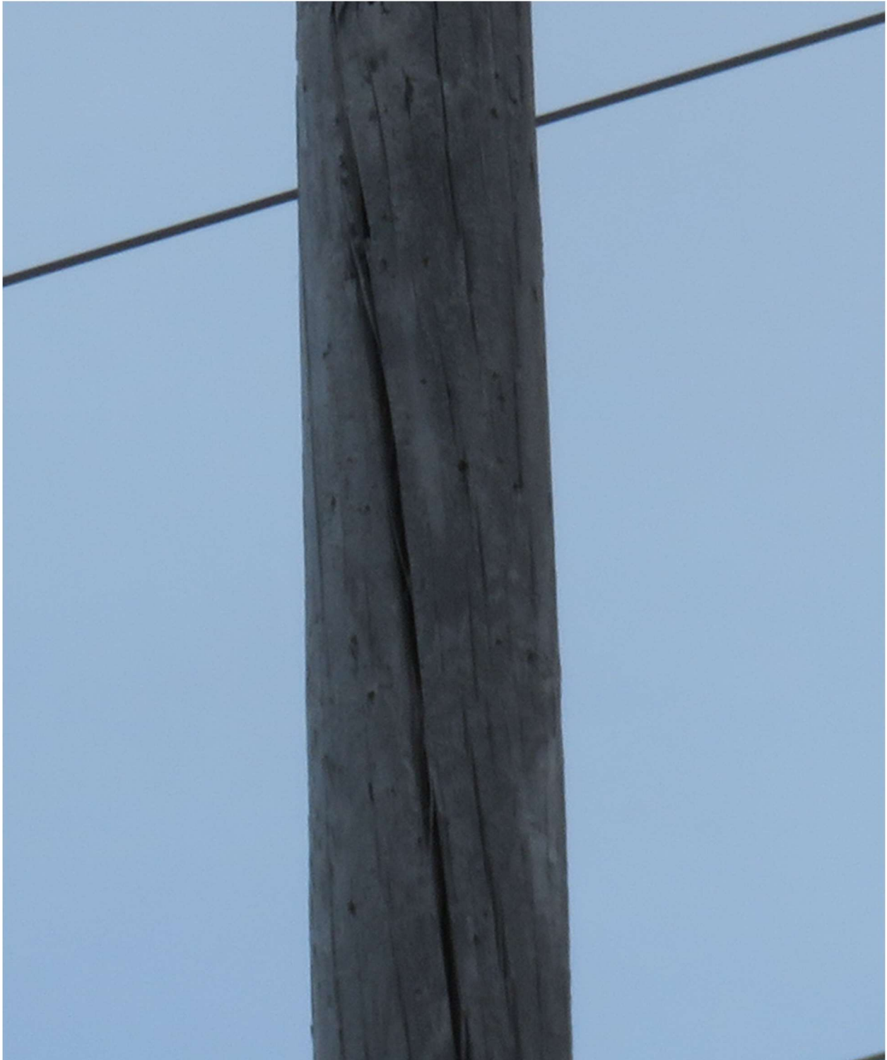
Figure B-7 – Large Split through Pole, Hollow.
