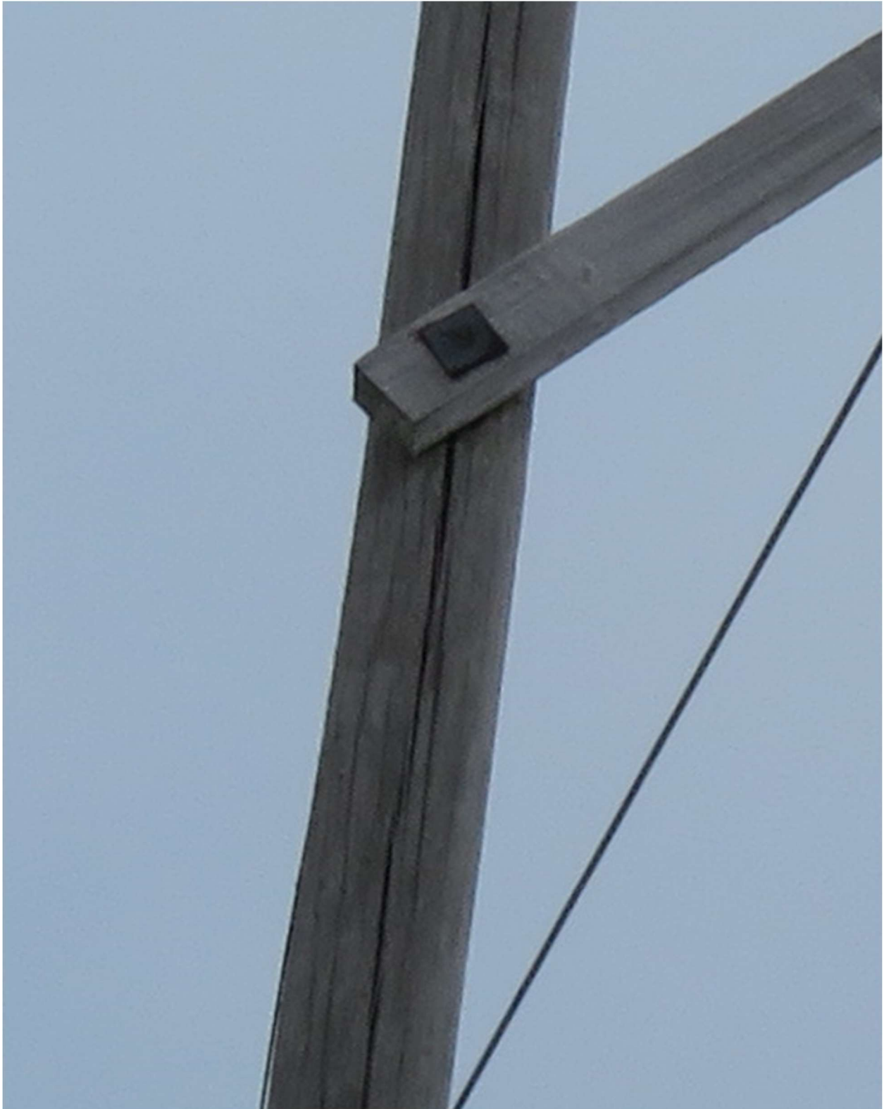
Figure B-4 – Large Split through Cross-Brace Bolt Locations.
