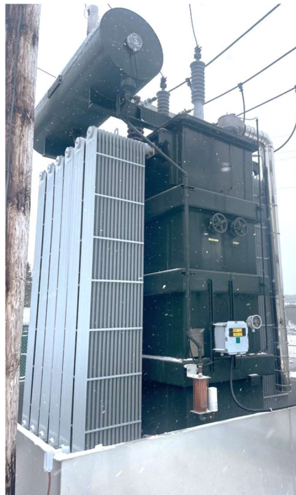
Figure E-6: Power Transformer MOP-T1.
