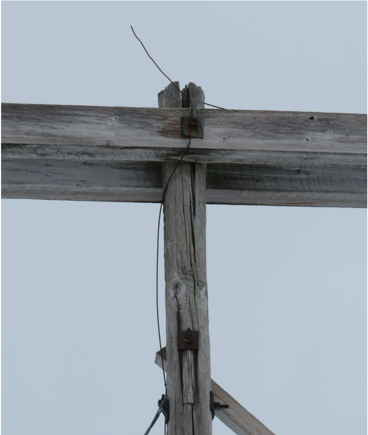
Figure B-2 – Cracked Pole Top and Splits through Cross Brace Bolts.
